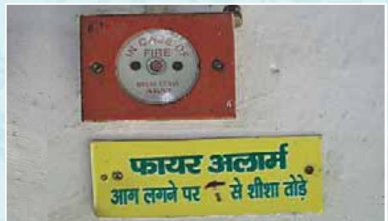
Emergency Fire Alarm Point
